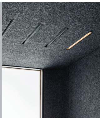
Efficient ventilation and lighting
